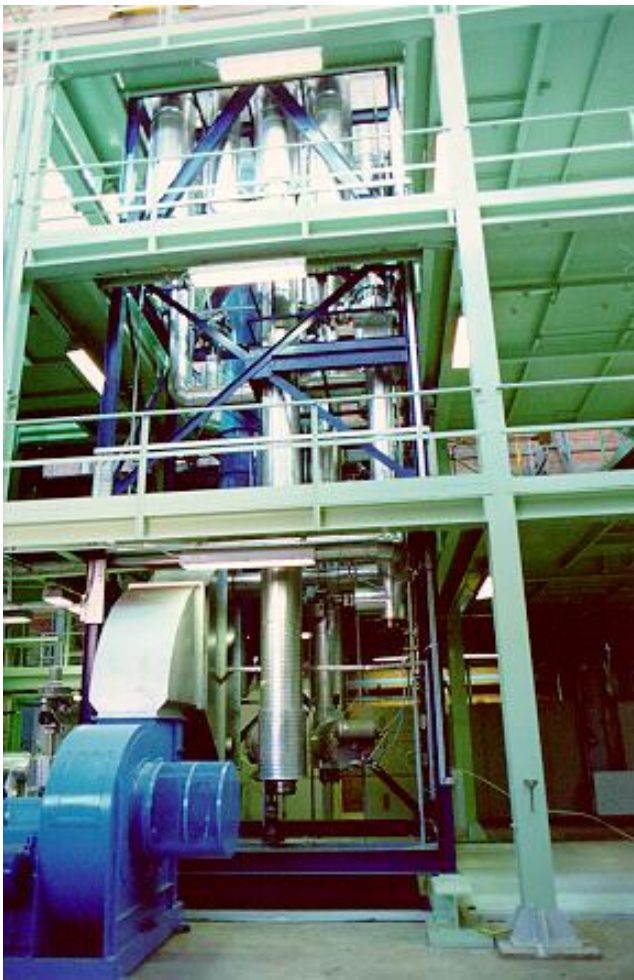
Fig. 1 – HeFus3 - European Blanket Test Facility
